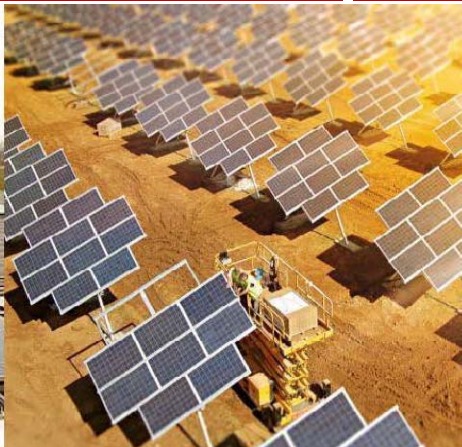
15MW Project in Mahora, Spain
