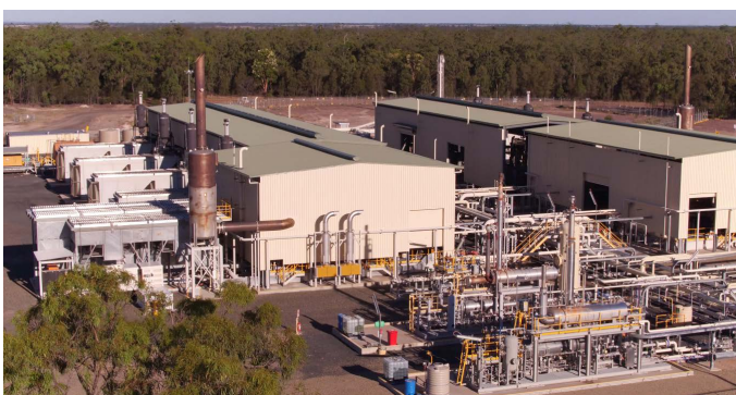
Daandine Power Station
