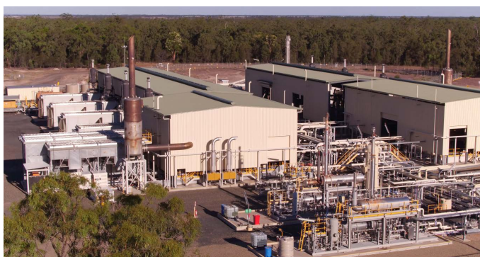
Daandine Power Station
